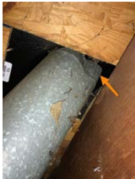
Stove Exhaust Duct
