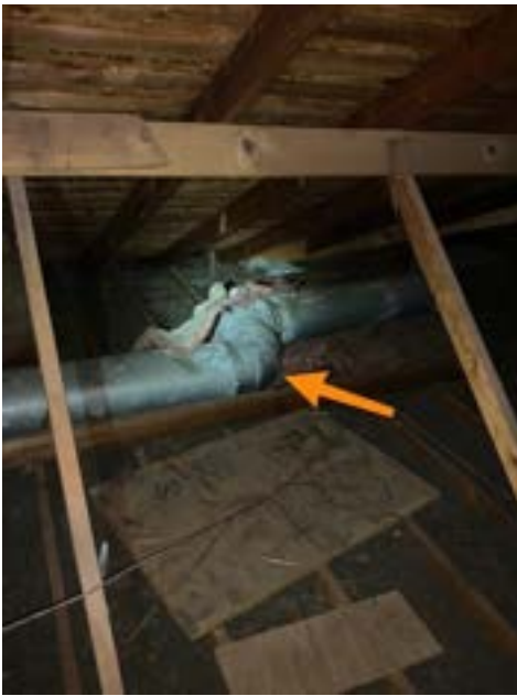
Return Duct Insulation
