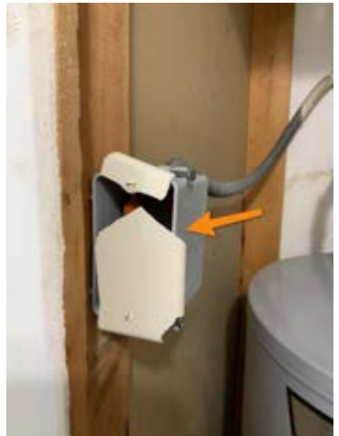
Water Heater Junction Box
