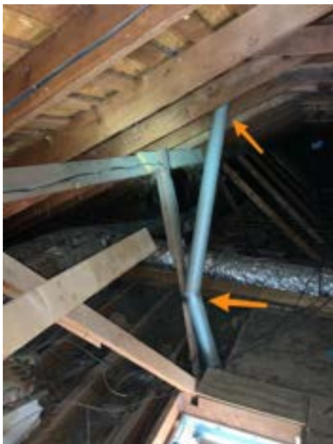
Stove Exhaust Duct
