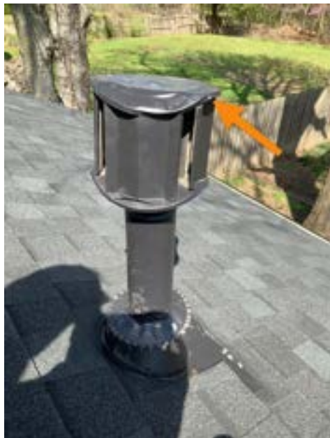
Water Heater Vent
