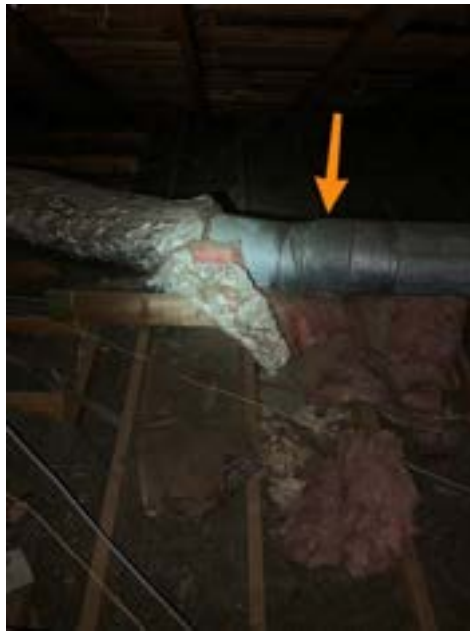
Return Duct Insulation
