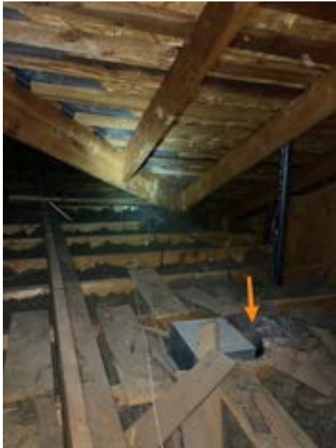
Primary Bathroom Exhaust Fan
