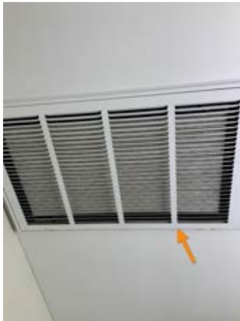
Return Air Ducts
