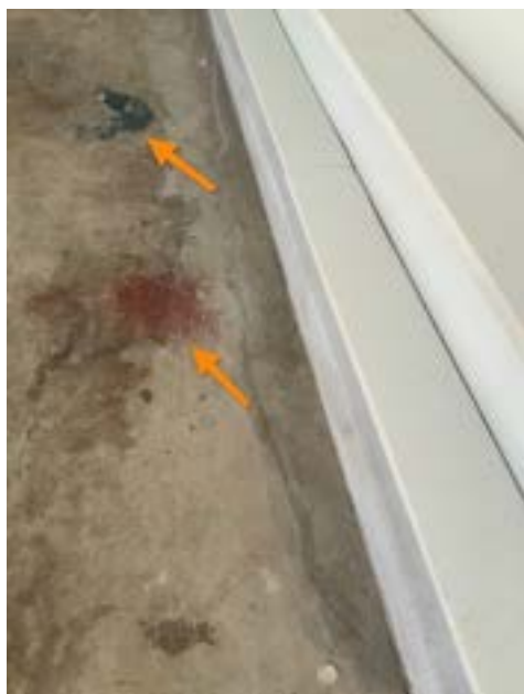
Garage Floor Staining
