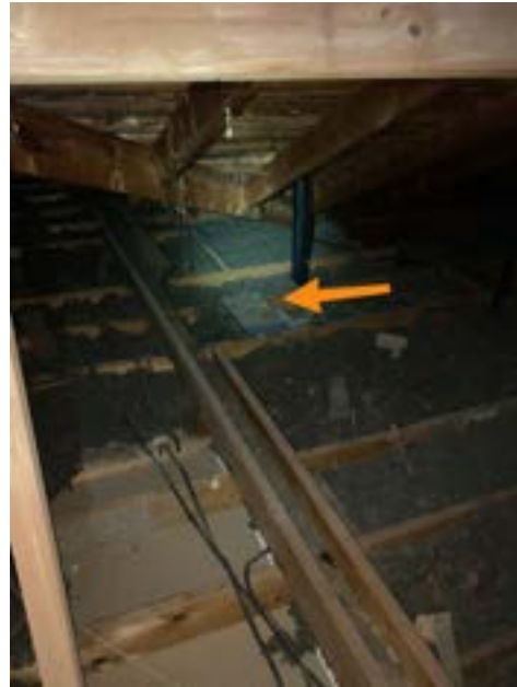
Second Bathroom Exhaust Fan
