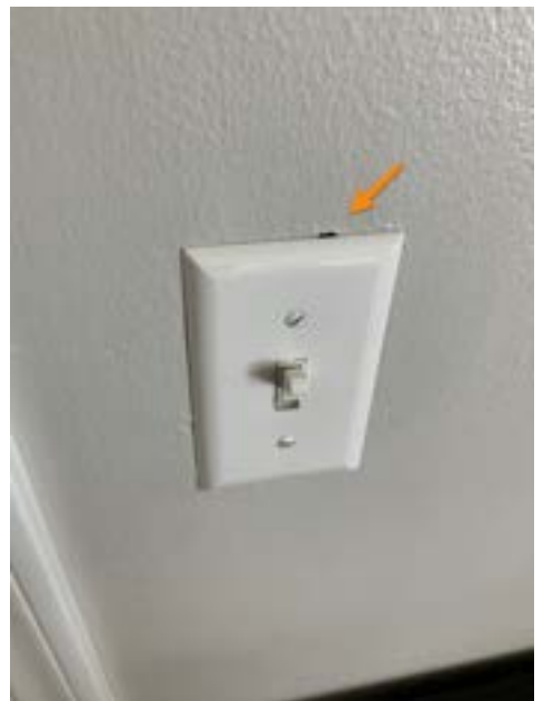
Dining Room Light Switch
