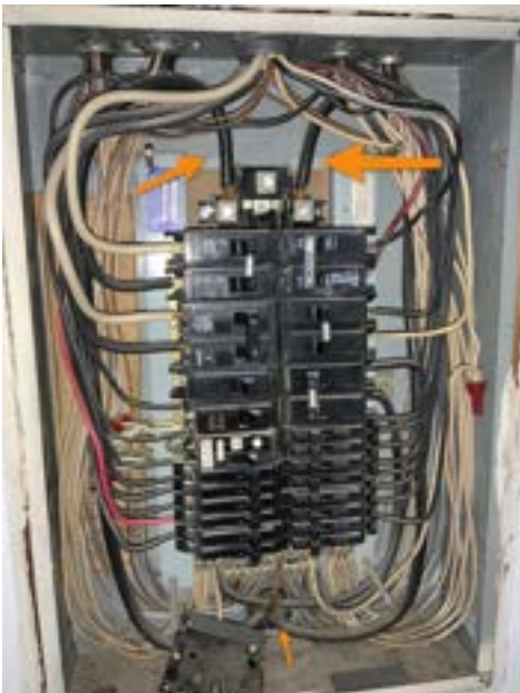
Entrance Conductors 2 AWG
